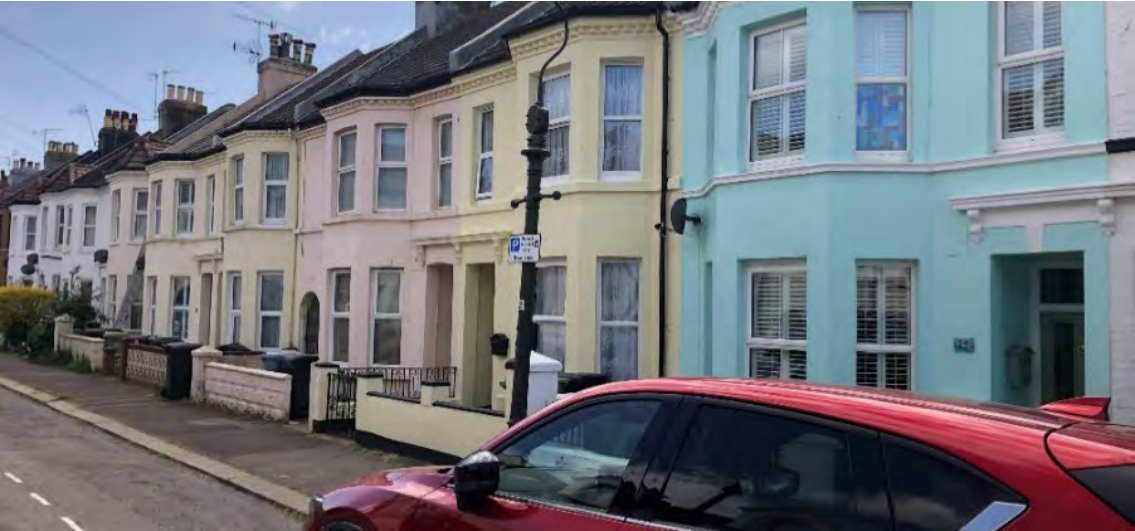
Figure 6: Photo of inappropriate PVCu casement windows
